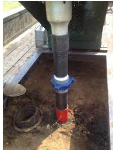
Figure 9 Well Head Enclosure
