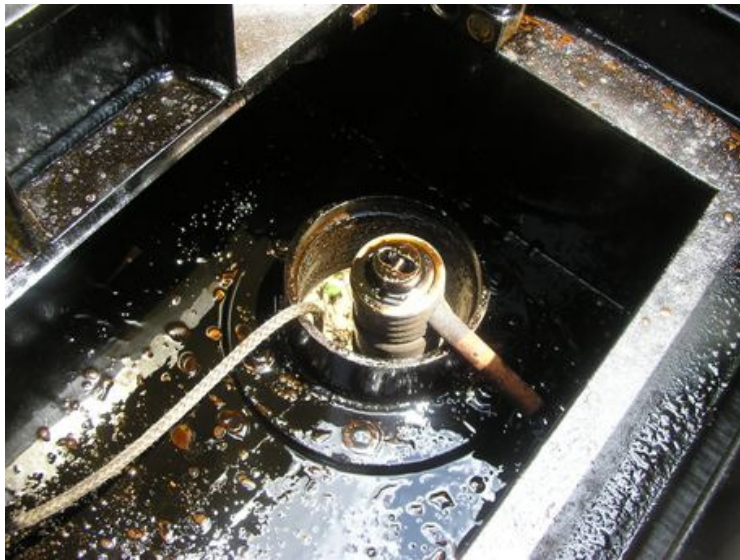
Figure 18 Dutchman attached to Bucket Head sitting on upper side of Well Head Flange
